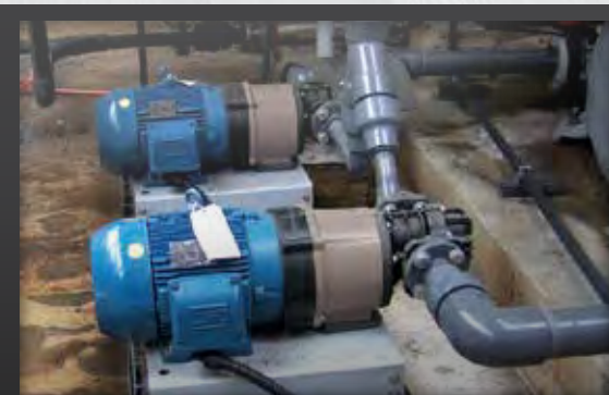
CMD pumps (main and redundant) metering industrial water treatment chemicals.
