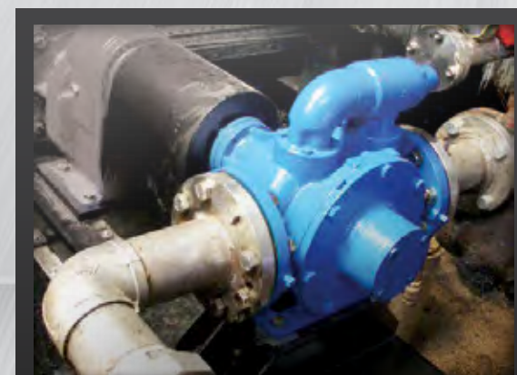
LVP series pumping water for emulsions.
