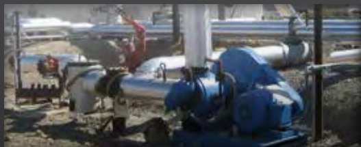
Jacketed pump blending asphalt at terminal.
