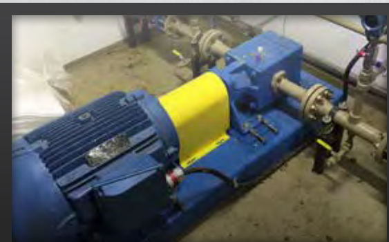
Pipeline booster pump in the Bakken Shale Formation.
